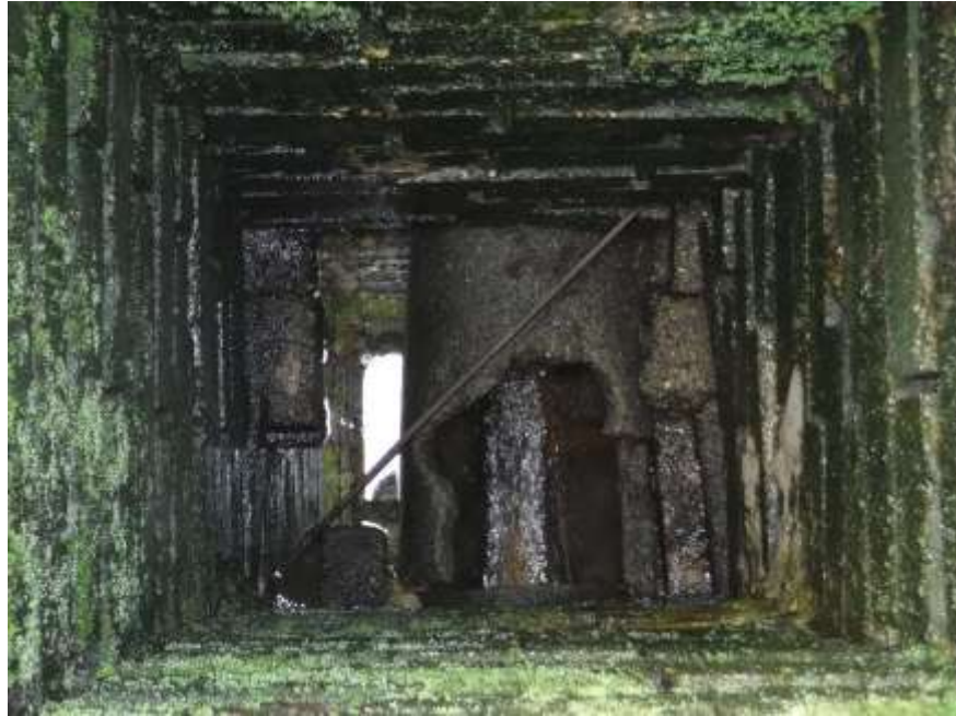
Image 5: Concrete pipe conveys flows through this CB
