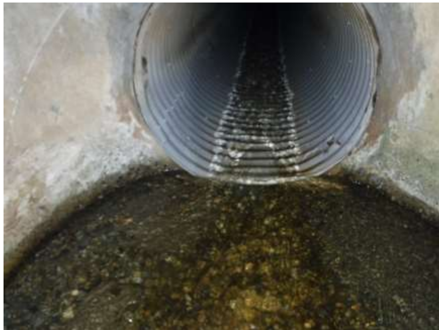
Image 10: flows outlet the CB via a 30" corrugated aluminum pipe
